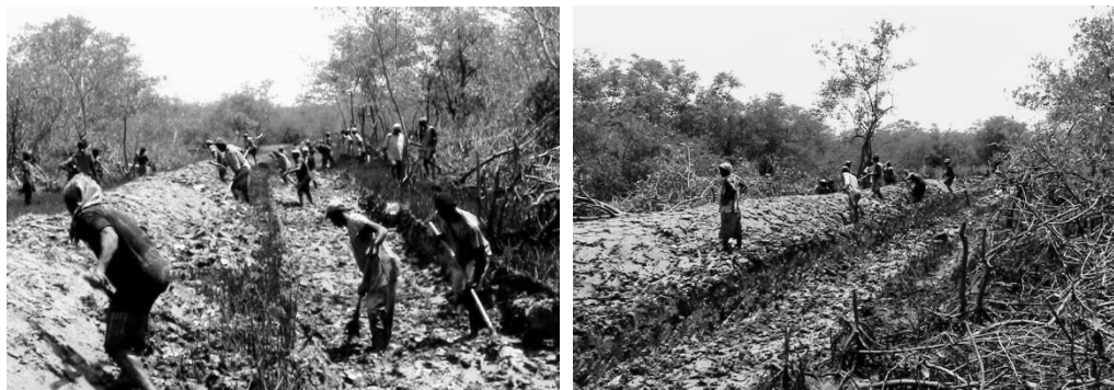
Figure 18- Construction of a main dike in Cantanhez in 2013 (Photos by Ana Luisa Luz).
