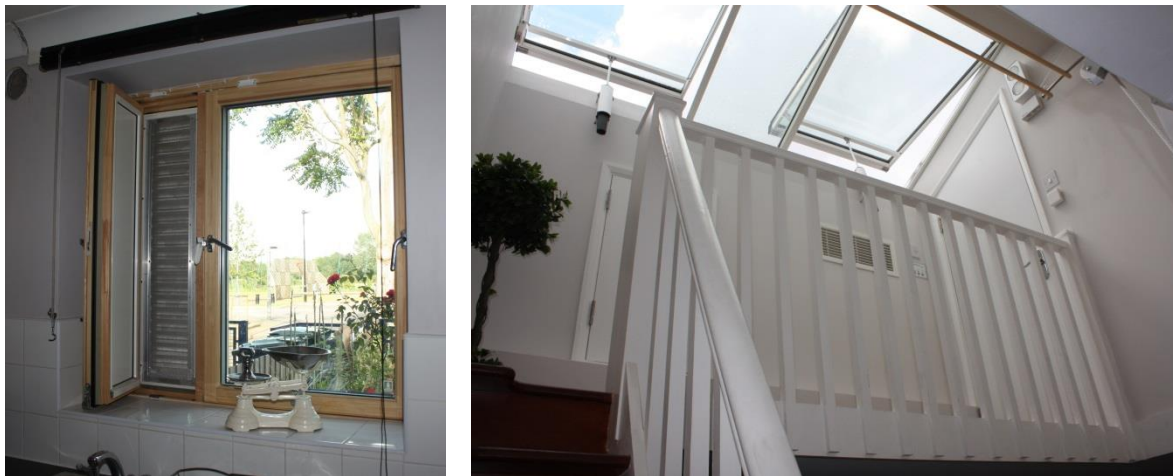
Figure 6 Modern house triple glazed windows with side ventilation panels (left) and automated roof-lights (right)
