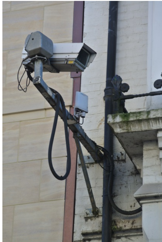
Fig. 7 CCTV in public space – Oxford
