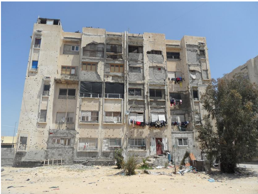
Figure 2.11: Partially damaged housing units in a five-storey apartment building that is still inhabited despite being targeted in Khan Younis, the Gaza Strip. Source: Salem Al Qudwa, 2013.
