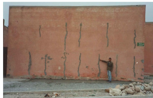
Figure 9. The pattern of vertical cracks identified on the external rammed earth walls of the houses in Mostefa Ben Brahim.
