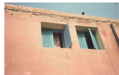
Figure 12. Vulnerability of rendering at the top of an external wall of a rammed earth house in Mostefa Ben Brahim, showing spalling of the rendering.
