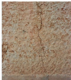
Figure 8. A vertical crack running across the full height of a wall of a rammed earth house in Mostefa Ben Brahim. Note the crack passing through the filled holes of the shuttering crosspieces.
