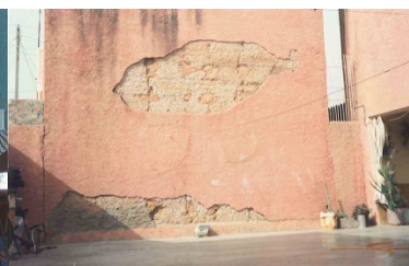
Figure 11. Vulnerability of the roughcast rendering used for the rammed earth houses in Mostefa Ben Brahim. Note the vertical cracks on the wall and black patches at the top of the wall.
