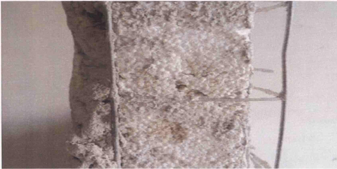
Figure 4.7: Closer view of partly sprayed EPS Panel meshed with steel connectors ( Location: CITEC Abuja, photographed by the author ).
