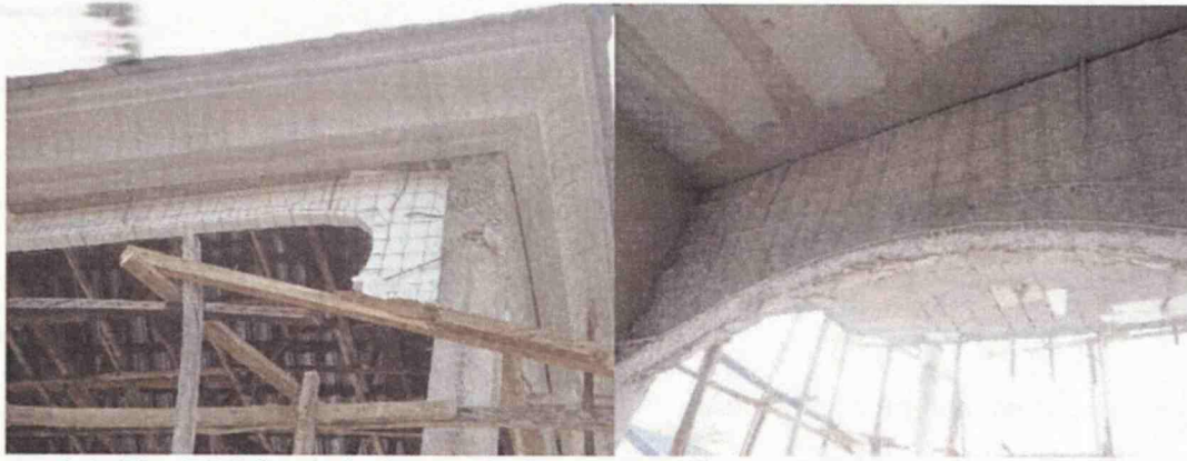
Figure 4.4: The EPS fascia before and after cement/fine and sharp sand spray ( Location: CITEC Abuja, photographed by the author ).
