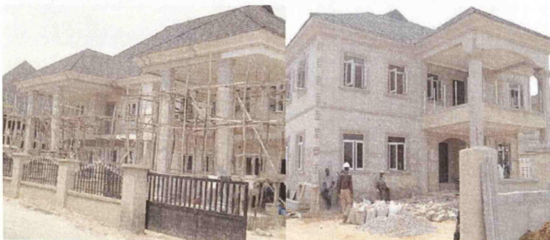
Figure 4.11: Fully cement plastered EPS houses ( Location: CITEC Abuja, photographed by the author ).
