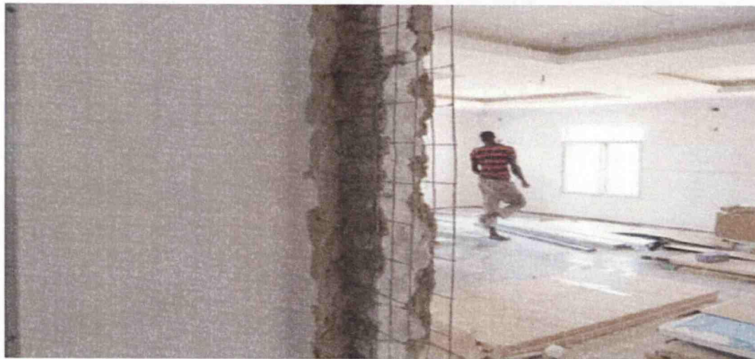
Figure 4.10: Internal view of a partly finished EPS house ( Location: CITEC Abuja, photographed by the author ).
