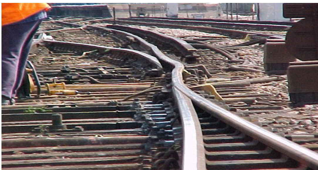
Figure 29: Track buckling risk contributor to derailment accidents
