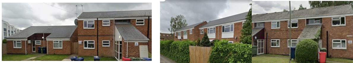
Figure 2. Samples of bungalows and flat façades with cavity wall insulation upgrades (left) and flats with no cavity wall insulation upgrades (right).
