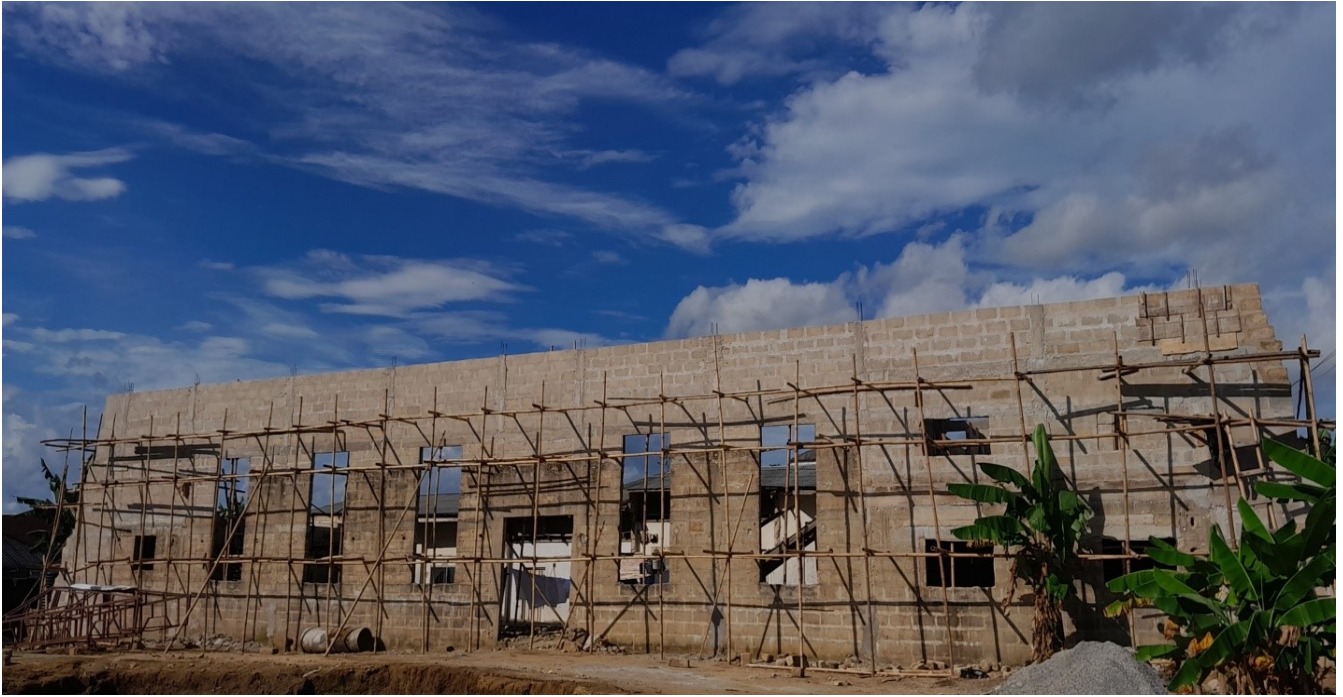
Figure 42 Wilfred Ukpong, VOF Foundation frontal view of the building construction, Eket, Nigeria, 2022
