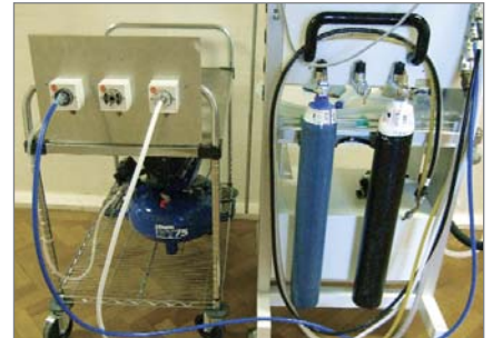
Figure 3 Anaesthetic machine pipeline probes connected to sockets
