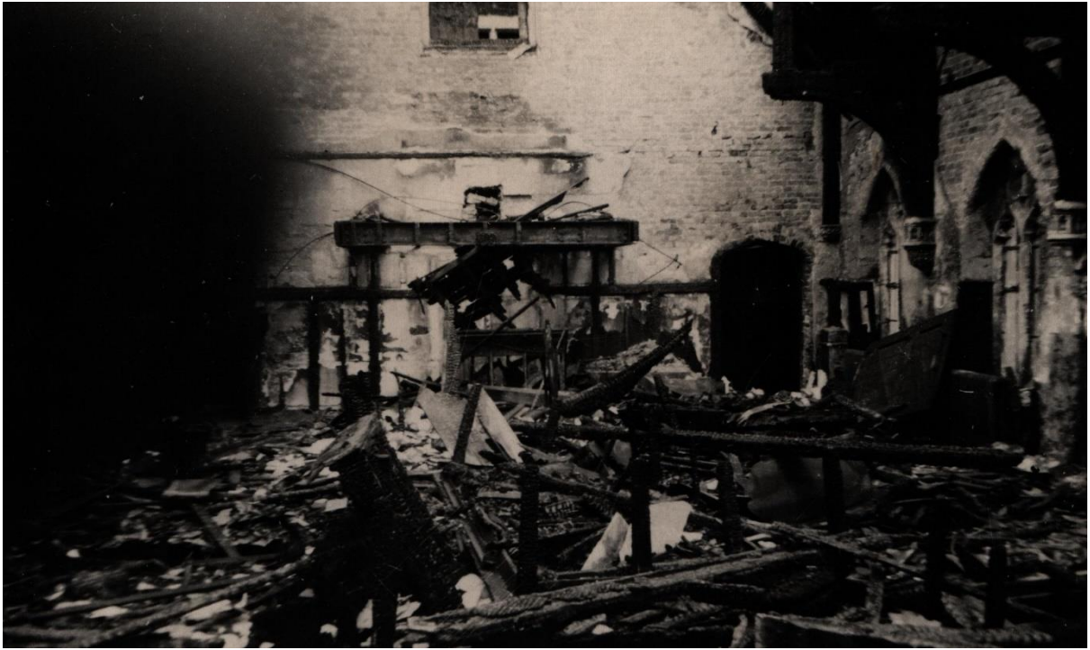
Image 16: Bomb damage to the Dining Hall, 1944.
