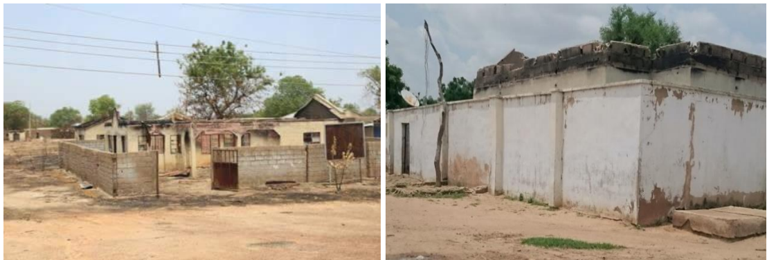
Figure 7.1a: Post-conflict condition of cement block houses in Buni Yadi
