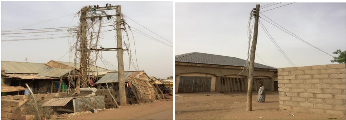
Figure 7.7a: Vandalised electricity infrastructure after the conflict in Bunia Yadi
