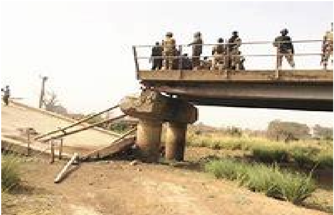
Figure 7.5a: Damaged bridge in Buni Yadi after conflict.
